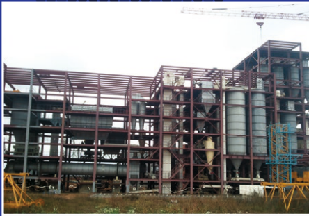
GYPSUM PLASTER PLANTS
